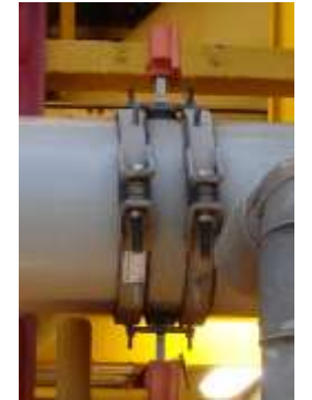
Permasense sensors clamped, to avoid welding (Courtesy NAM)
