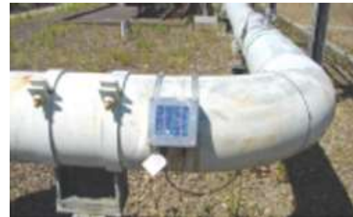
HOIS field trial with ClampOn CEM system at Shell UK gas plant
